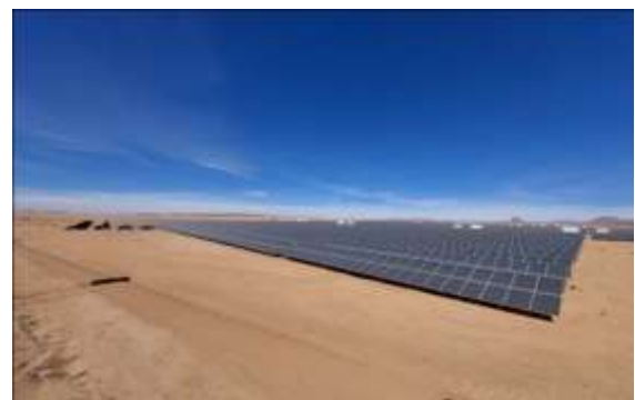
Figure 1. Photovoltaic Power Plant in Tamanrasset, Southern Algeria
