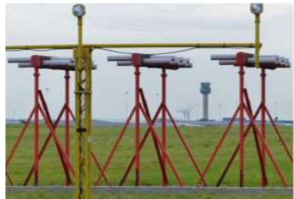
Figure 11: ILS systems ground antennas
